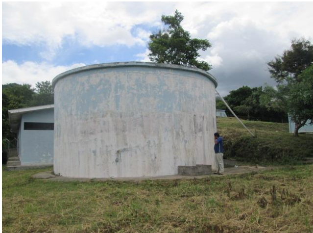
Tanque grande circular
