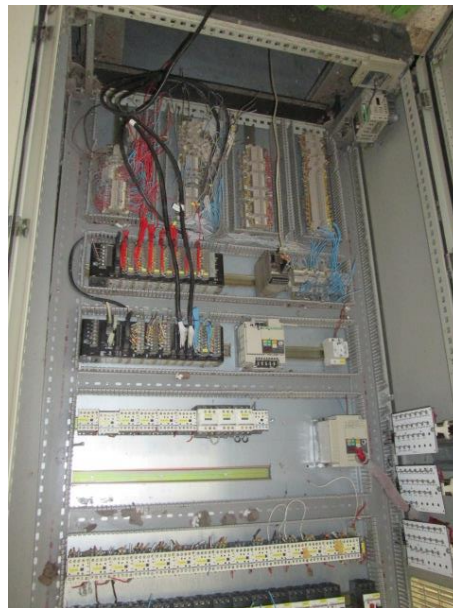
Vista interior panel de control principal
